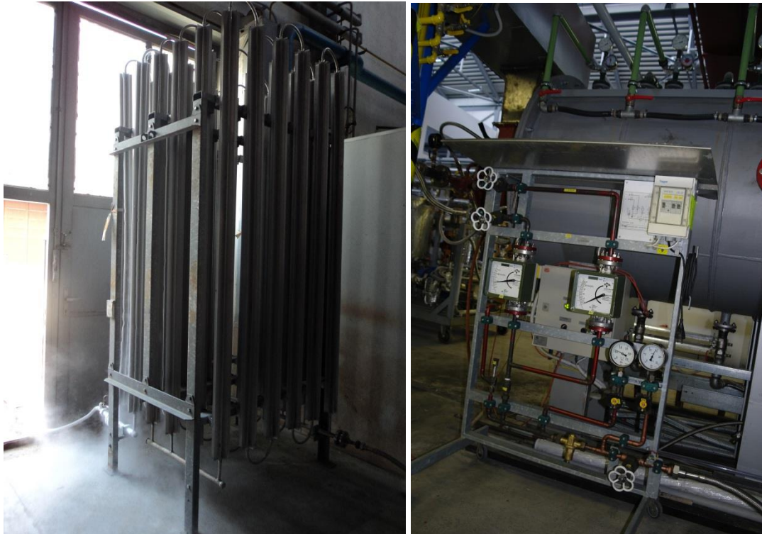
Figure 6.5 – (a) The evaporator and (b) the measuring panel.
