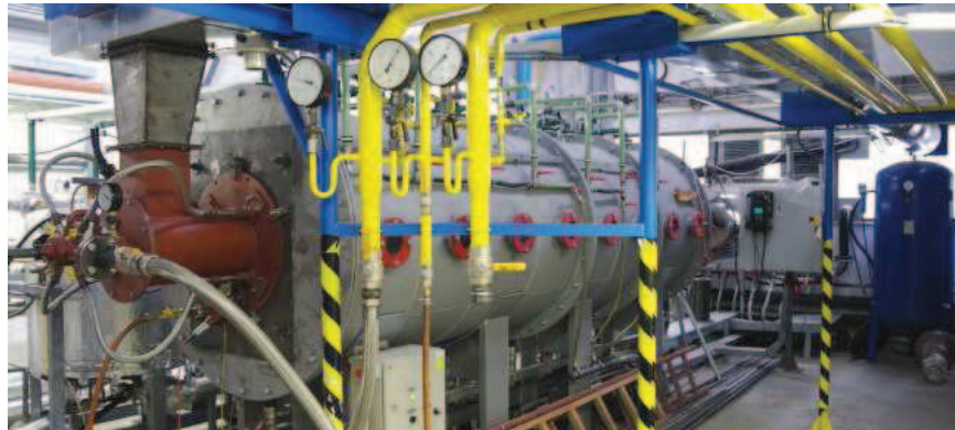
Figure 34: Burner test chamber [13]
